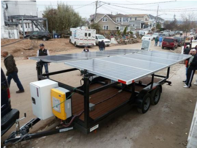
Figure 4: Solar generators were used to help New Yorkers after Superstorm Sandy. Credit: Consolidated Solar [16]
