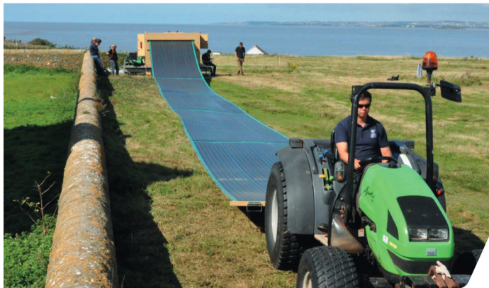
Figure 2: Rapid Roll unfurling solar arrays like a carpet from behind a truck [2]
